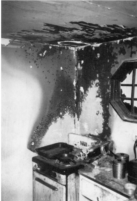
FIGURE 6.2.11 Clean Burn on Wall Surface.
