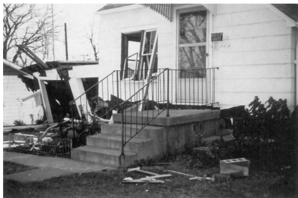
FIGURE 21.3.1 Low-Order Damage in a Dwelling.
