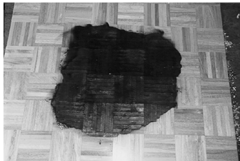
FIGURE 6.3.7.8.3(c) “Pool-Shaped” Burn Pattern Produced by a Cardboard Box Burning on an Oak Parquet Floor.
