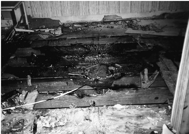
FIGURE 6.3.7.12 Saddle Burn in a Floor Joist.
