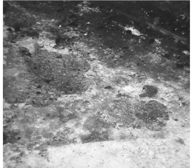
FIGURE 6.2.5.1 Spalled Concrete Floor.
