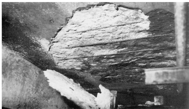
FIGURE 6.2.5.1.3 Spalling on Ceiling.
